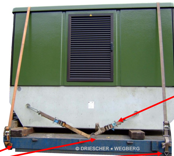
Station mit Betonfundament Station with concrete foundation
